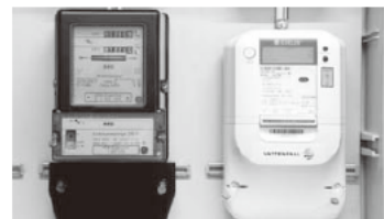
MI-003: Electricity meters
